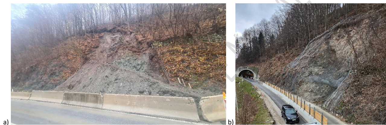
Figure 1: Initial situation of the landslide hazard on the E652 near Tržič before (a) and after (b) the urgent remedial measures (Foto: DRI).
