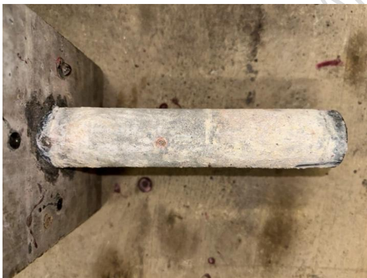
Figure 6: Expansive zinc-oxide development on the surface of a zinc-clad dowel.
